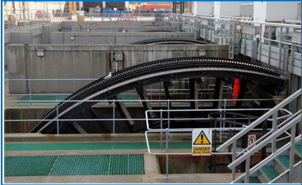
Figure 2.1 The four drum screens at Sizewell B
